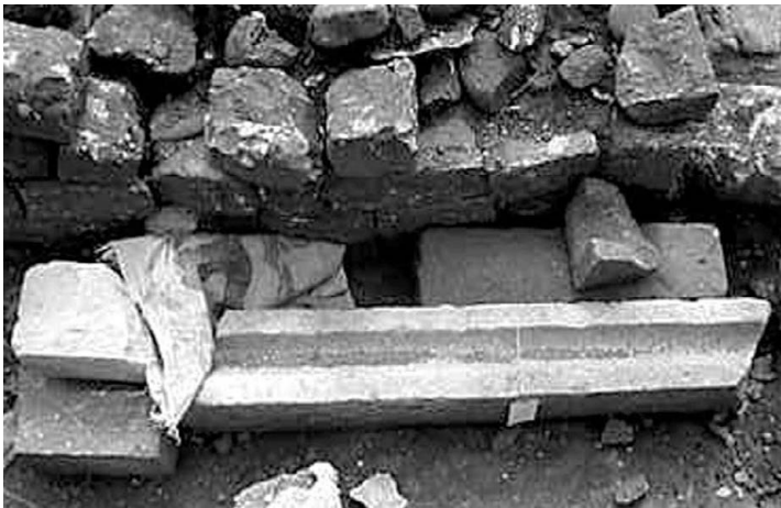
Figure 3-21. Fallen drain stone.
