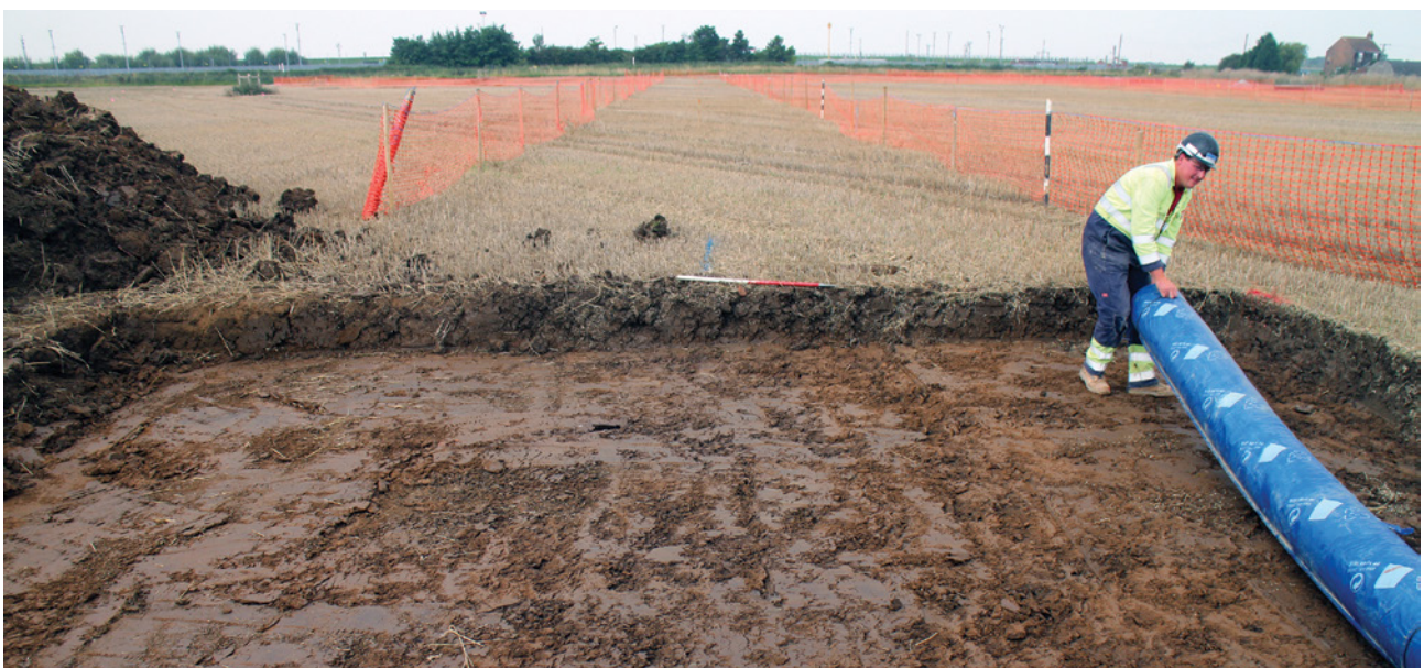
Plate 2: The watching brief at the Paull AGI in progress, with the estuarine landscape in the background, looking north-east
